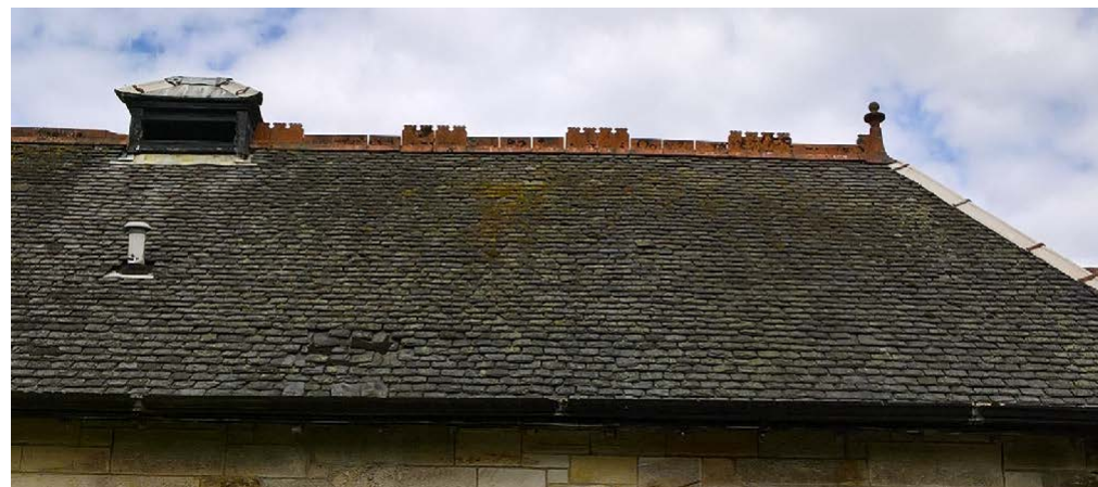
Slates missing and slipped
