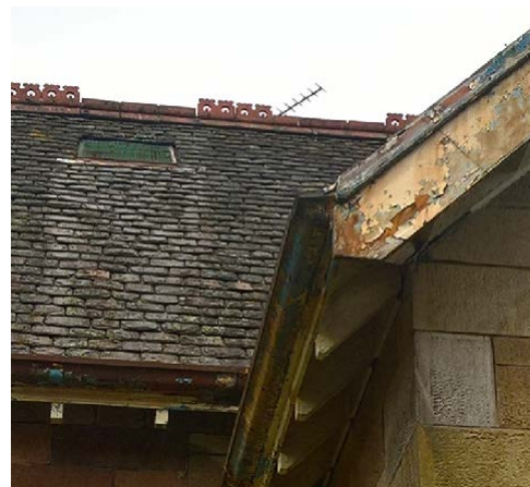
Blocked and corroded guttering
