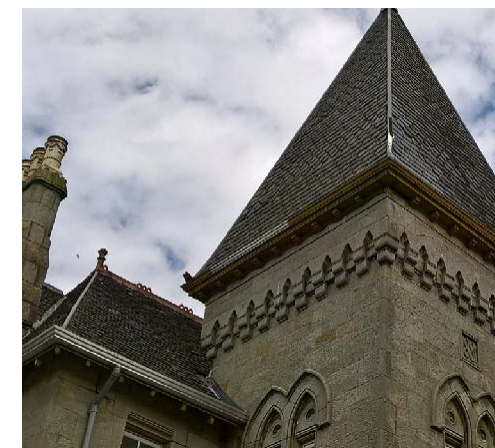
Roof flashing missing - Spanish slates in use
